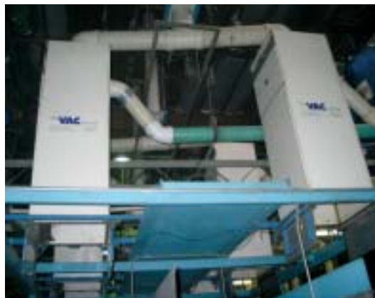
Mission's Phoenix plant uses a vacuum system to move textiles from soil sorting to the wash aisle.
