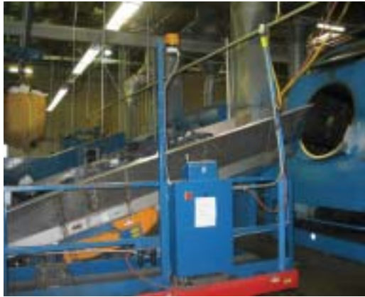
Industrial items are transferred from one side of the wash aisle to the other using a semi-automatic shuttle system.
