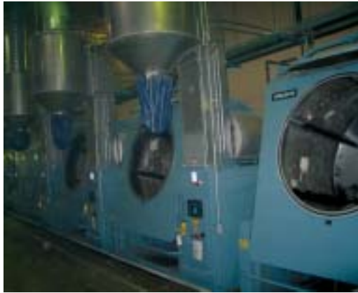
CLM dryers are also used on the linen side of Mission's Phoenix operation.
