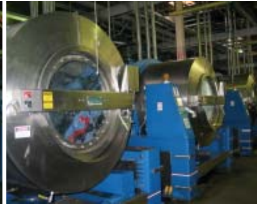
Industrial garments seen here are being processed in a Brim 450 lb. washer.
