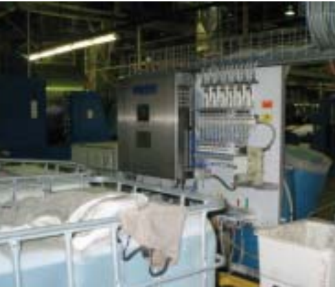
The plant uses several technologies to increase efficiencies, including this Dober chemical-injection system.
